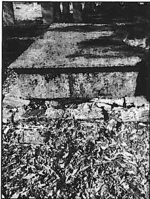
Figure 25. Broken base of vault.
